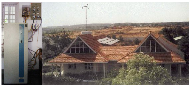
Figure 11. Photovoltaic UPS and array
